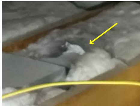
Blocked by insulation
