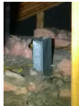
Kitchen cooktop hood fan vent pipe terminates just above ceiling level into the attic. Vent pipe needs to be connectd to the exterior to expel cooking gases (air/grease/moisture).
