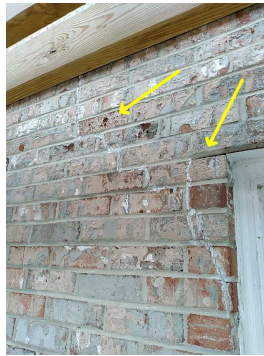
Common settlement cracking observed
