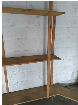
Typical settlement cracking
