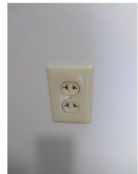
2 prong outlet. Unable to test
