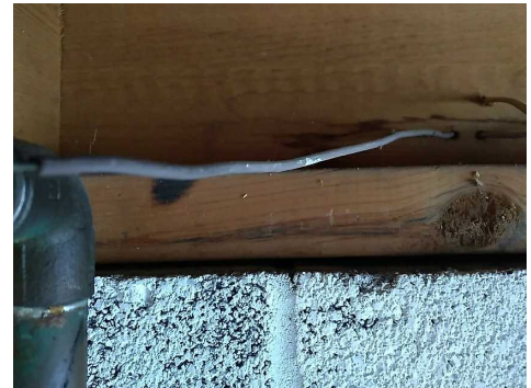
No sill plate flashing
