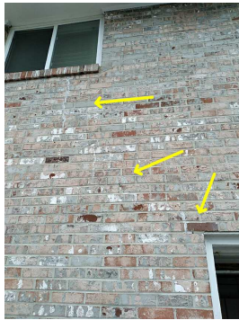
Common settlement cracking observed
