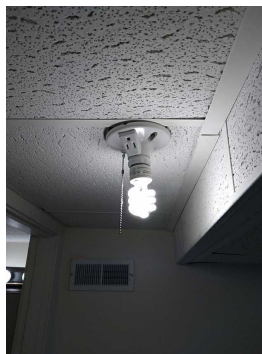
Missing fixture globe
